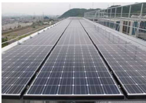
Solar panels (Minase Research Institute)
