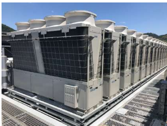
Module-type heat pump chiller (Minase Research Institute)
