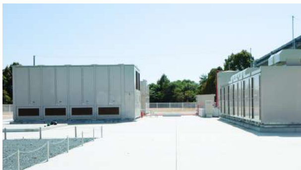
Large-capacity power storage system (Yamaguchi Plant)
